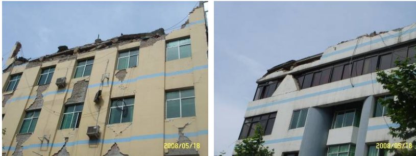
Fig. 4. Failure of the parapet wall
