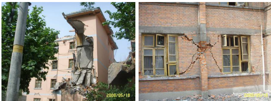
Fig. 1. Through diagonal or X-shape cracks on the wall
