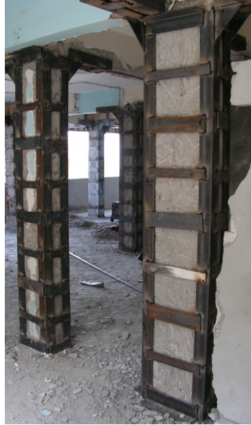
Fig. 13. Steel jacking applied to RC columns (Photo by Dr. Ali Haydar Kayhan)
