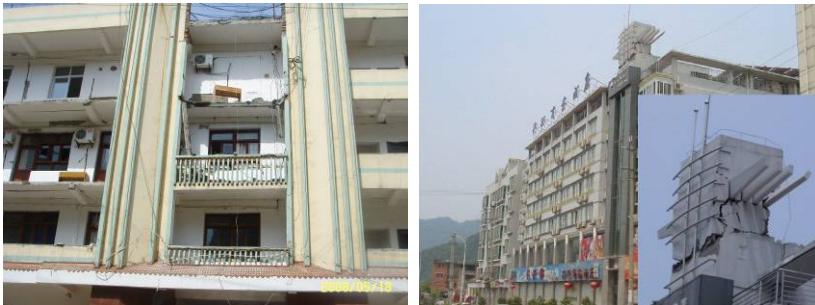
Fig. 5. Falling of the corridor fence and horizontal crack of the protruding member
