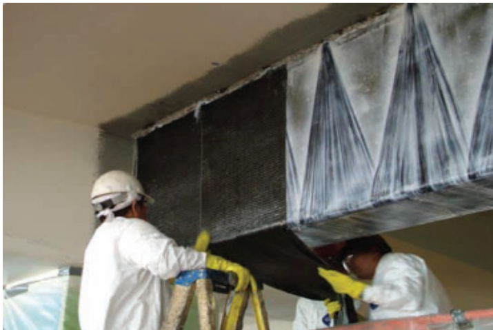
Fig. 14. FRP confinement of a beam (reprinted with the permission of FYFE Europe)
