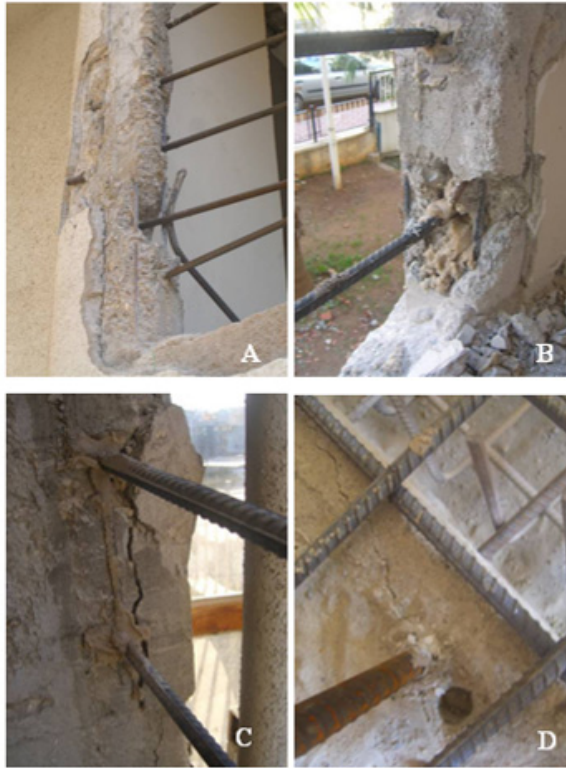
Fig. 18. Poorly implemented anchor examples (A, B: anchors implemented on defective surfaces; C: Anchor implemented near a crack; D: Anchor fracturing the concrete during the tensile test)
