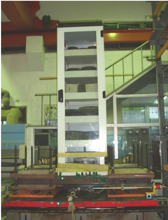
Fig. 31. Critical equipment isolated with DO-FPS isolators
