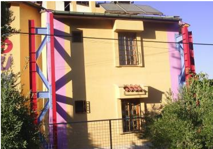
Fig. 11. Buttress type external steel shear wall (Photo by Dr. Yavuz Selim Tama)
